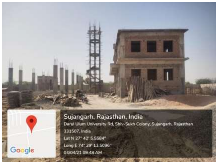
Figure 10.4B: STP-2&3 located at the same place under construction in Sujangarh Rural (Capacity of each plant is 1.5 MLD)
