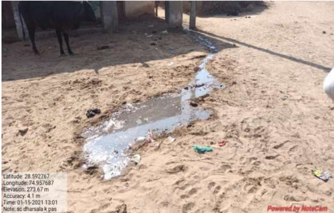
Figure 15.9E: Current status of stagnation of Grey wastewater on Main Road ( Aam Rasta ) (Community Sock pit/ Leach Pit and Individual Sock Pit for individual household is required)
