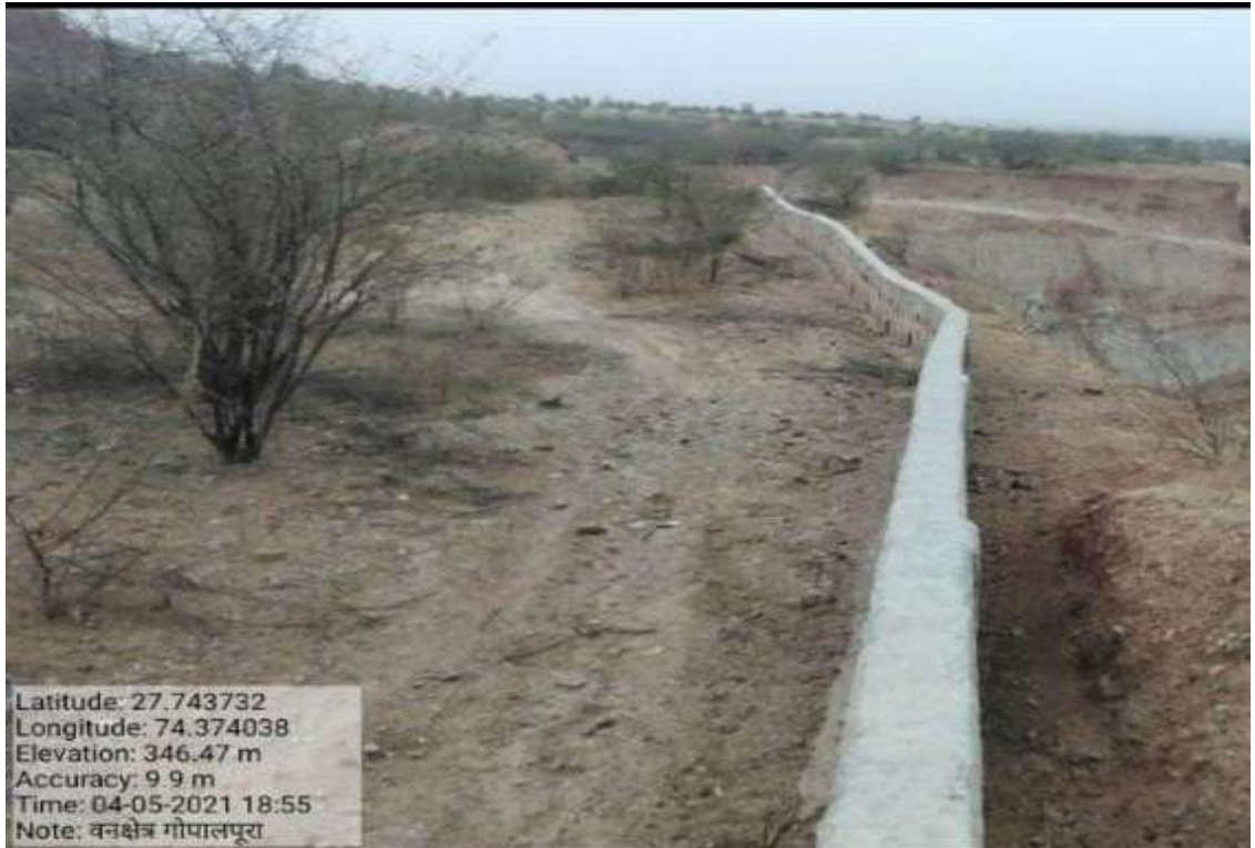
Figure 14.4: Control of illegal mining in Sujangarh range by constructing pucca boundary wall in forest area
